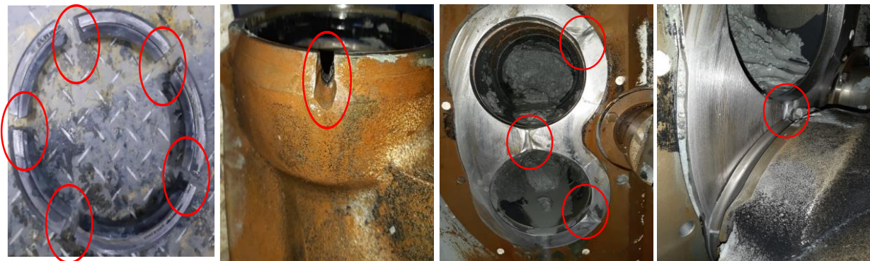
(a) Cutting ring (b) Seal (c) Insert ring (d) Housing lining Fig. 11 Damage of cutting ring and seal of rock valve
